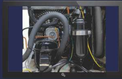
1 TON COOLING SYSTEM SMALL COOLING SYSTEM
