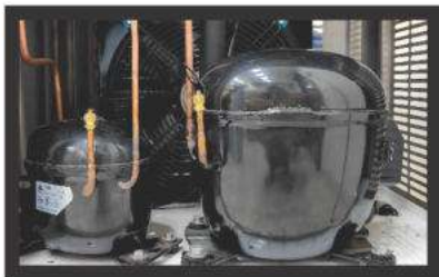
1 TON COOLING SYSTEM COMPRESSOR
