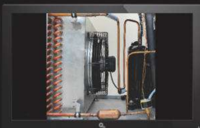
1.5 TON COOLING SYSTEM COMPRESSOR
