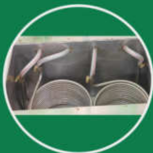
ICE STORAGE TANK
